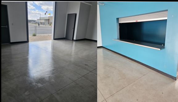
Pictures of the sealed floor in the HOM building; almost ready to go!
